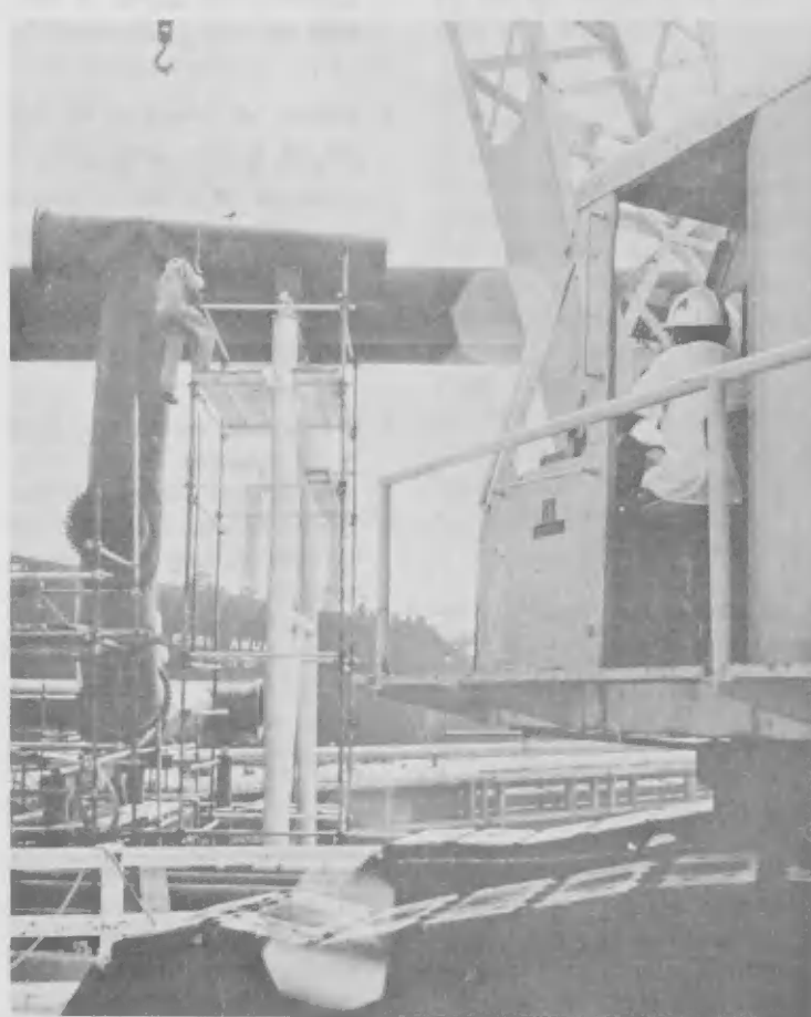
Equipment Operator P. Maduro here lifts a 36" T and elbow in place for welding near Finger Pier No. 3.
